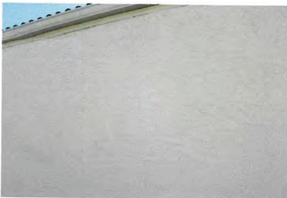
7 Stair step hairline cracking
