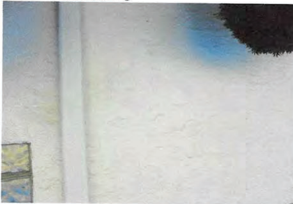
5 Vertical hairline cracks
