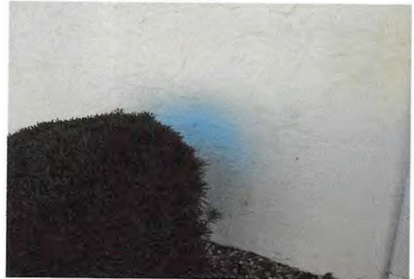
6 Vertical hairline cracks
