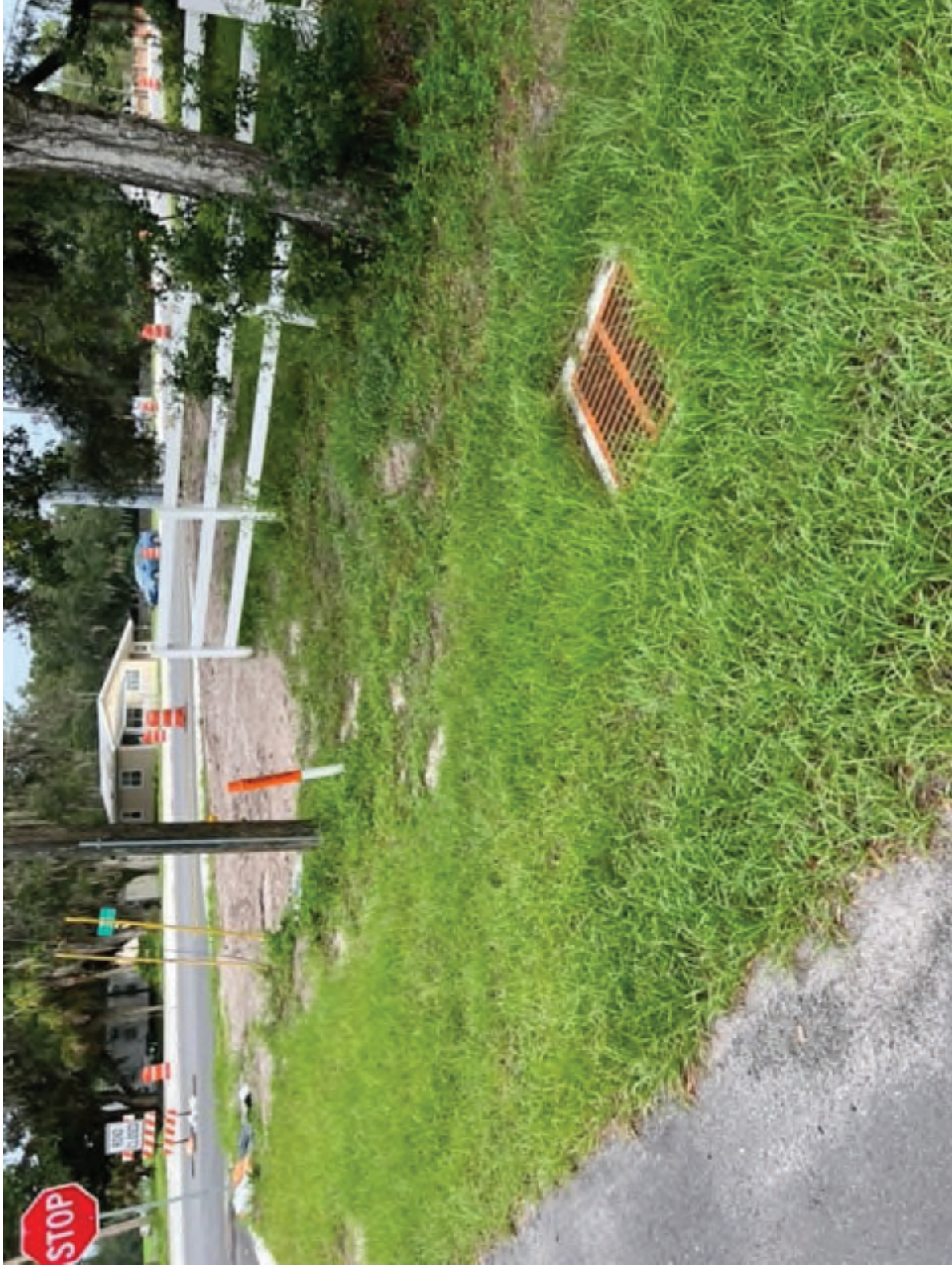
View of Myrtle Road facing West Near Intersection with Bell Shoals Emphasizing Stormwater Infrastructure South of Myrtle
