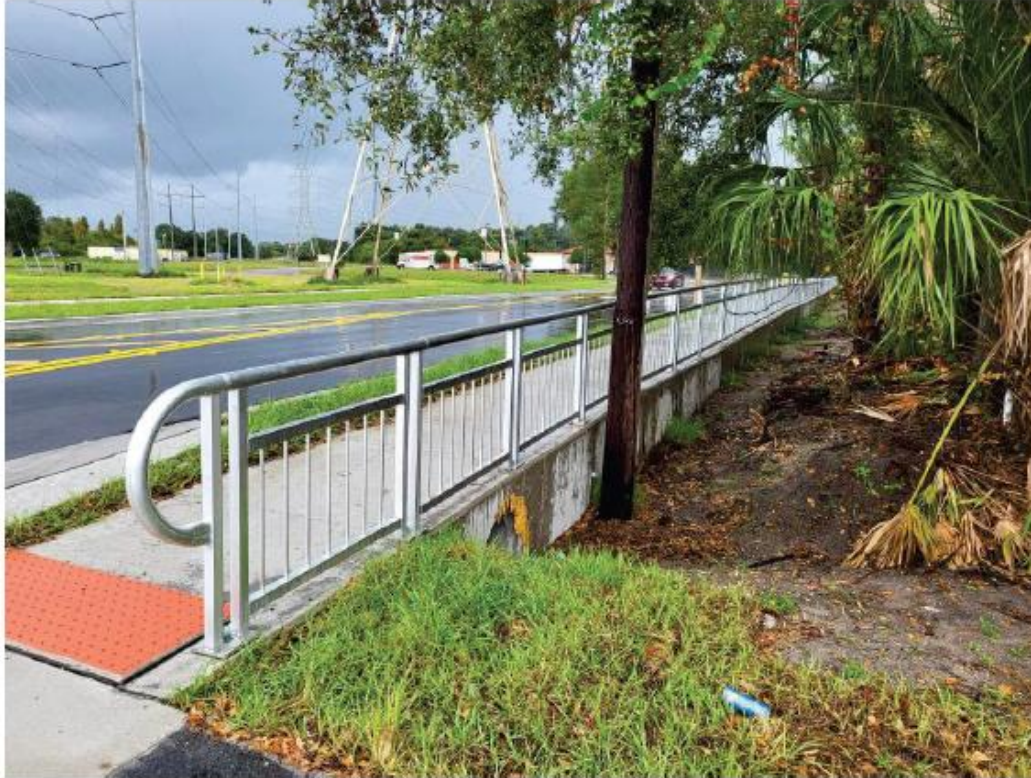
PHOTO OF NEWLY-CONSTRUCTED SECTION OF 86TH STREET – NOTE ELEVATION AND RETAINING WALL
