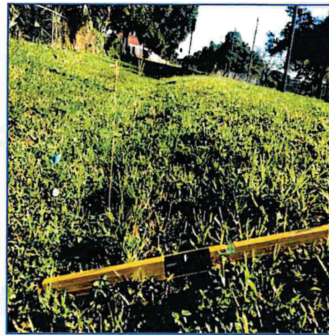
Photo 2 – Front Slope Greater than 1 to 4 to Become Steeper with Widening of Rural Typical Section
