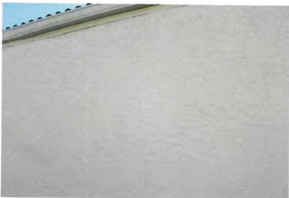
7 Stair step hairline cracking
