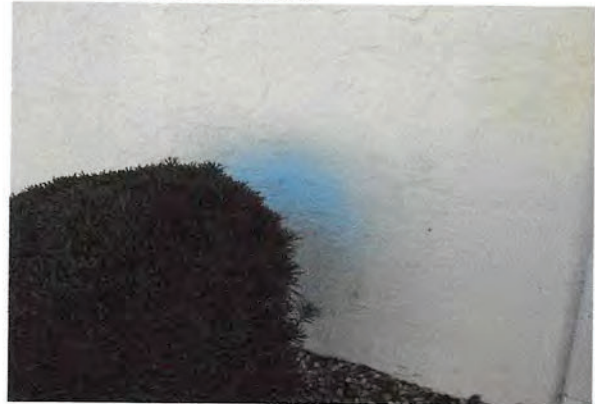
6 Vertical hairline cracks
